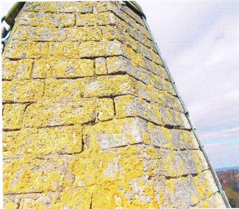
Open Joints 3.5m Down
